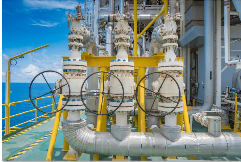
Fig. 3. Safety valve configuration on processing unit.
