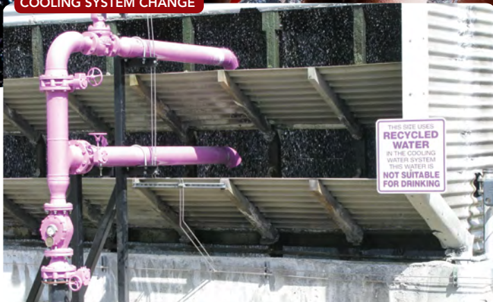
Figure 2. Santa Clara, Calif., hydrogen plant now uses recycled water as makeup for cooling system. Source: Air Products.
